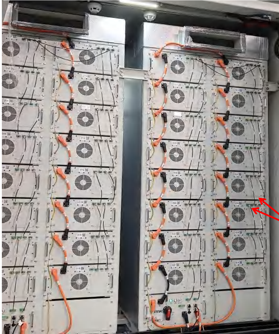
PACK: Communication and Fan Power Cables
