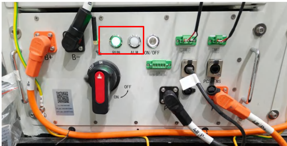
high voltage box power indicator
